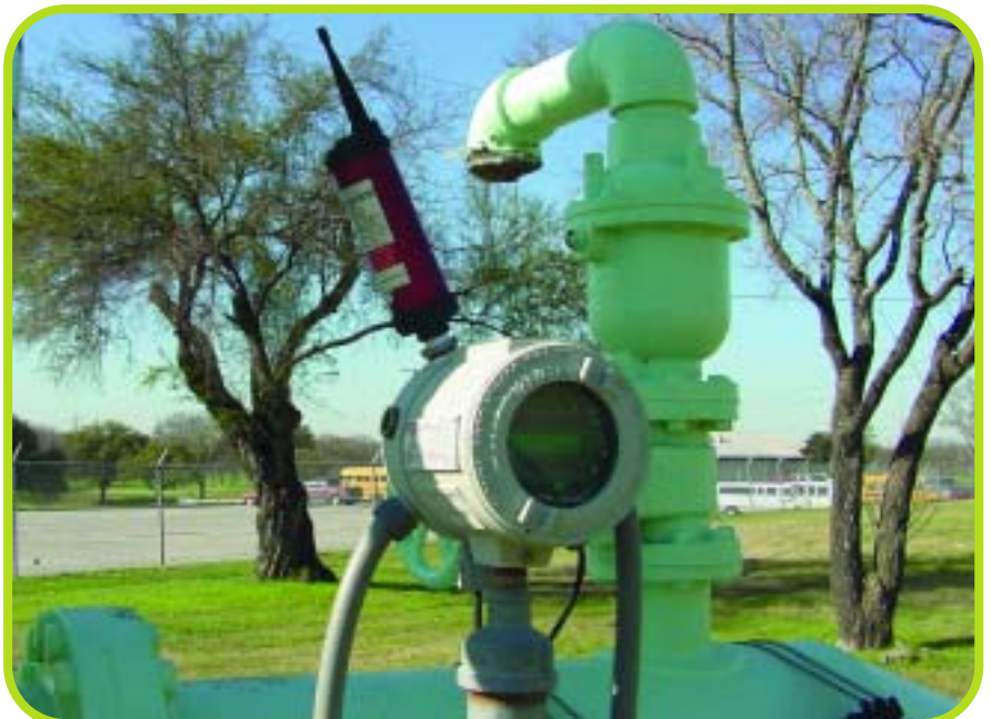
Radio attached to equipment outside the San Antonio Water System.
