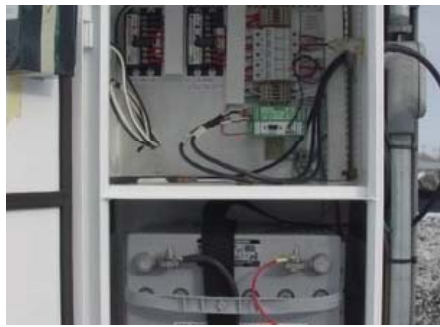
Solar Interference System (SIS) from Phoenix Contact provides wireless telemetry at remote tank monitoring site without an A.C. power source.
