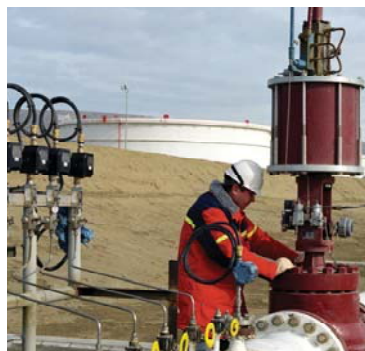
Remote monitoring at BP Refinery
