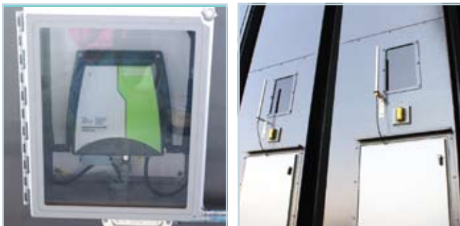
Ethernet radios with antennas monitor video from the stadium's kinetic wall
