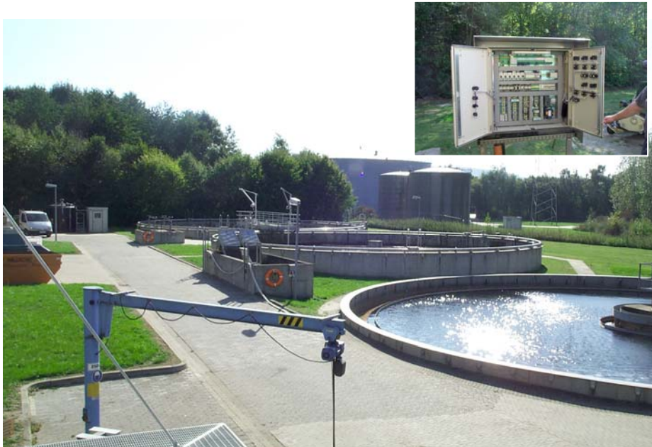
Porta Westfalica/Möllbergen sewage treatment plant
