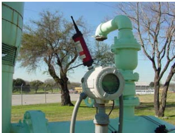
SAWS uses NIMA 4 conduit mount transmitters to communicate from several flow transmitters
